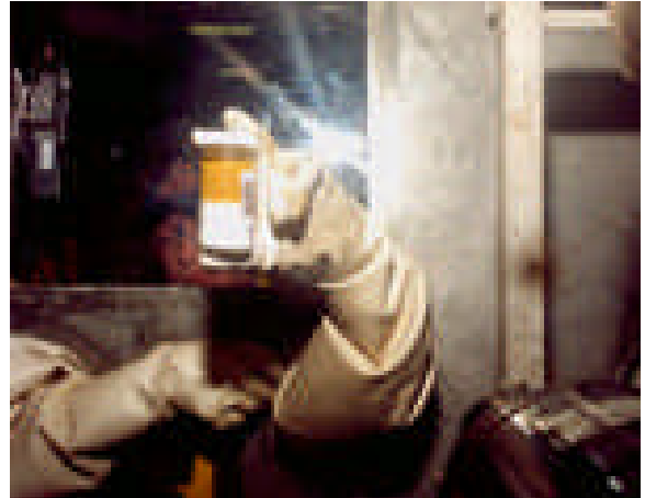
Nochar Demonstration Of Oil Stabilization After Nochar Was Introduced Into Waste Oil Inside Building 774.
